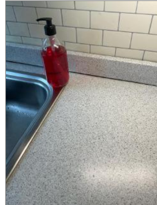
Photo - 15 Missing mastic joints
