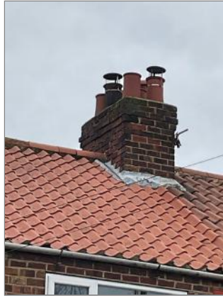
Photo - 4 Defective pointing
