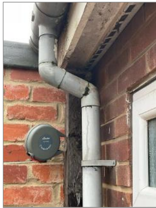
Photo - 7 Rainwater goods - defective joints
