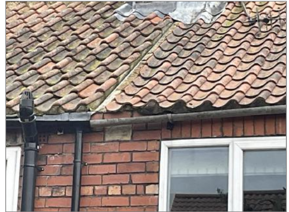
Photo - 6 Eaves - Defective pointing
