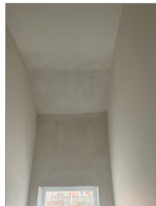
Photo - 11 Ceilings - Condensation & mould
