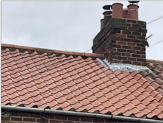
Photo - 5 Ridge - frost damage
