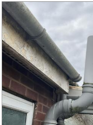
Photo - 9 Decorations - Defective
